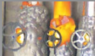
Thermal Fusion image of steam leaking from a pipe due to insufficient insulation
